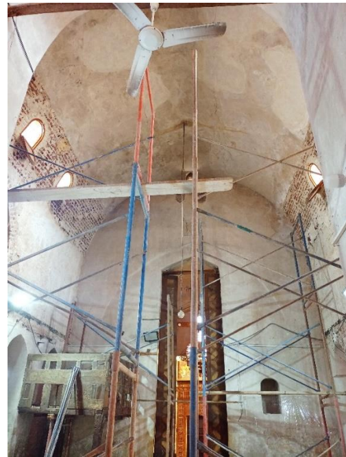
Figure 10. The effect of rain and floods on the church from the inside
